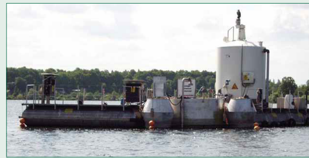
Deep-water ventilation system
